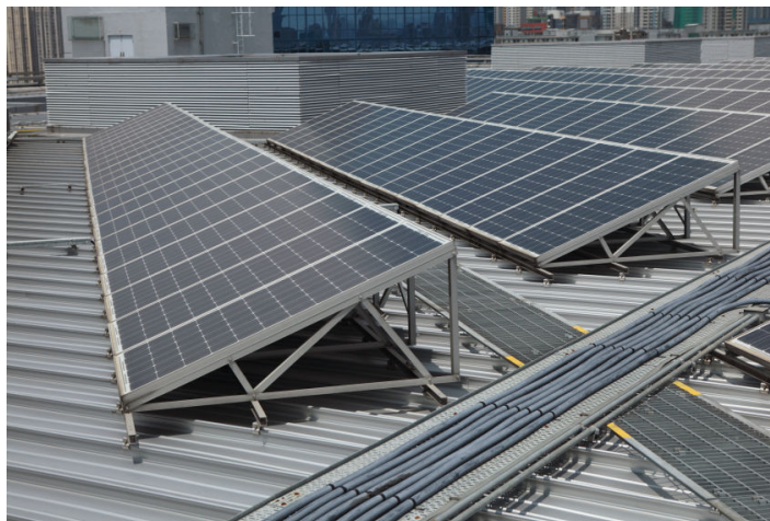
Solar Installation: A grid of solar panels connects to an inverter, which in turn communicates to a dataTaker data logger.
