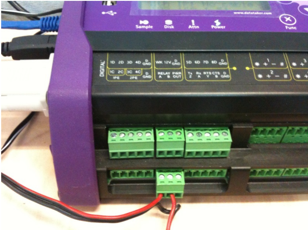
Figure 2 - Relay connection for the modem power cable
